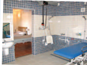
Specially equipped hygiene rooms
